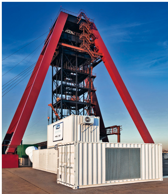
Fig. 7: Commissioning of ventilation system for number 2 shaft at the mine in Belarus
