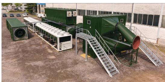
Fig. 8: Assembly of the ventilation system for the service shaft at the factory (from left to right: exhaust-air container, 2 air-cooled chillers, intake-air container with attached E-house container and 2 stacked cooler containers)
