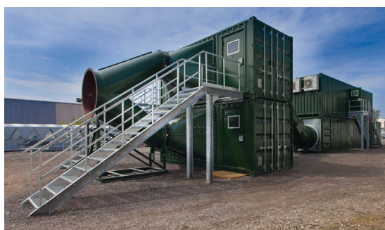
Fig. 9: Assembly at the factory viewed from a different angle (in foreground 2 cooler containers each with a 1,000 kW finned-tube air cooler)
