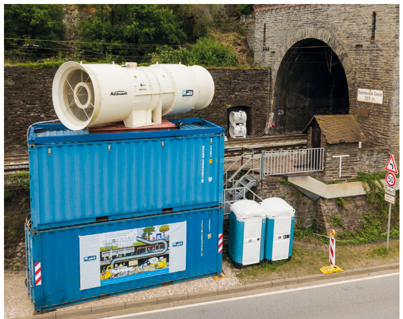
Fig. 2: Tunnel ventilation system during tunnel refurbishment
