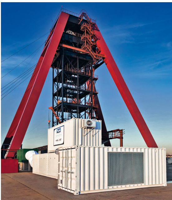
Fig. 1: Shaft ventilation plant
