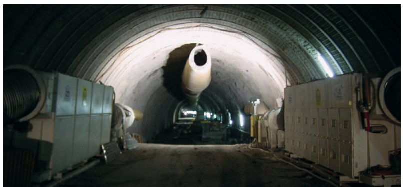
Fig. 3: Looking back from the tunnel face towards the fresh air duct and dedusting equipment
