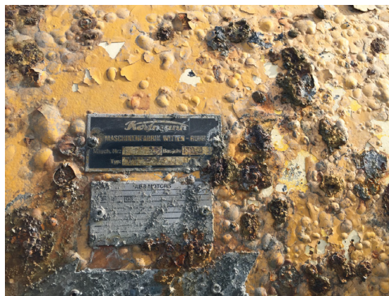
Fig. 17: Surface corrosion caused by moisture and salt-laden air
