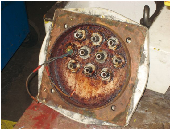
Fig. 18: Chemical corrosion inside a mine fan
