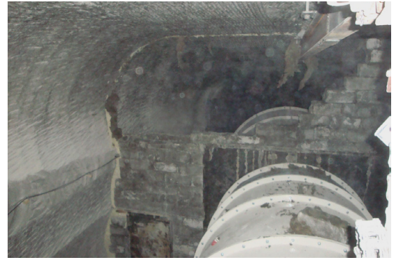
Fig. 4: Collapsed air screen
